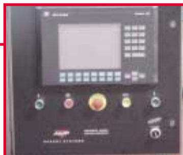
Operator Interface Panel
